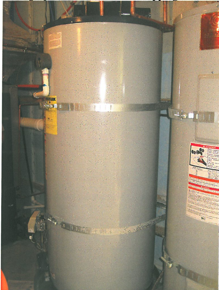
Photograph 8: Water heater strapping.
